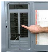
Look for tripped breakers or blown fuses
